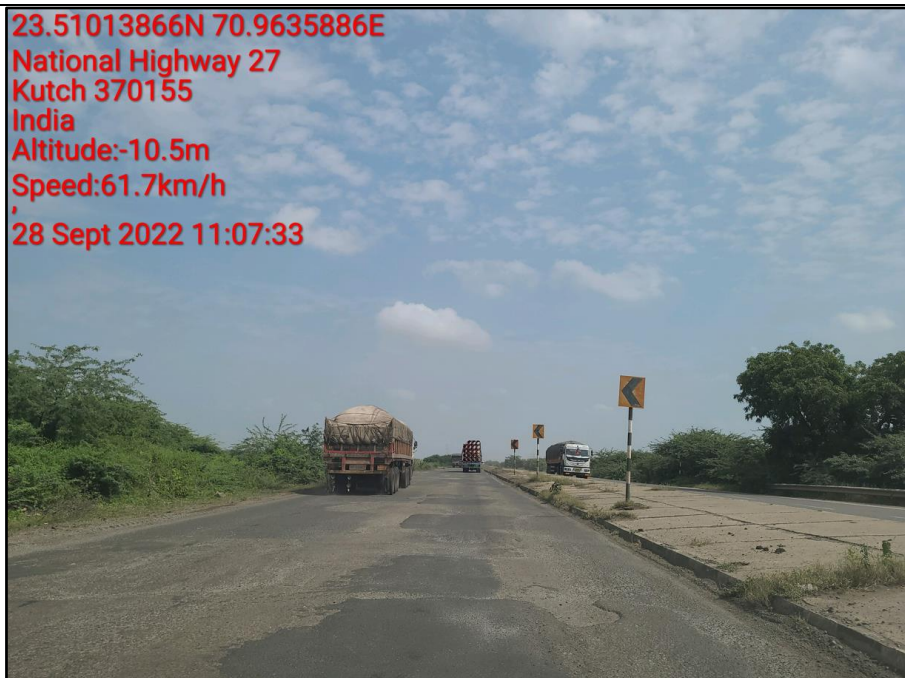
Figure 1-3 : Worn out wearing course of project road.
