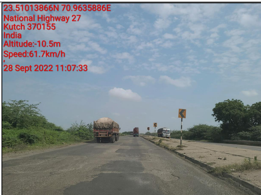
Figure 1-3 : Worn out wearing course of project road.
